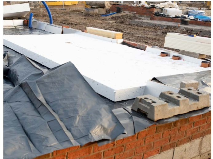
On modern construction sites, blocks of polystyrene form an insulating layer for new homes being built
